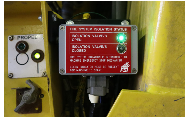
Fire System Isolation Status Panel
